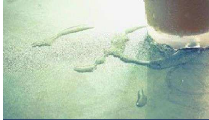
SURFACTANT LEACHING/WATER MARKS
